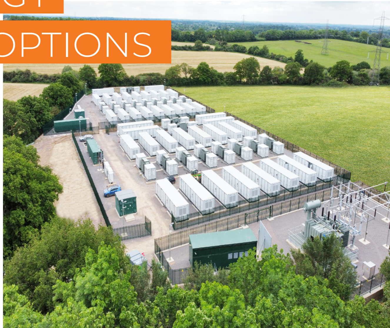
The largest unsubsidized grid-connected standalone battery storage plant in Europe: 100 MW/100 MWh Energy Storage plant at the 400 kV UK national grid substation in Minety, UK.
