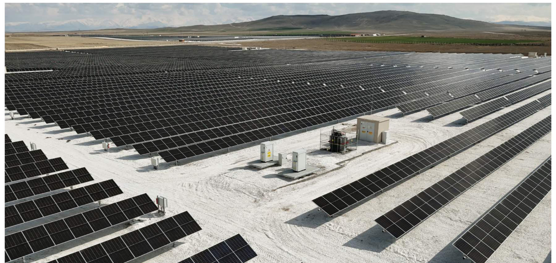
The 105 MW AC PV park is one of the largest in Turkey and was the first installation of the 1+X modular inverter solution in the country.
