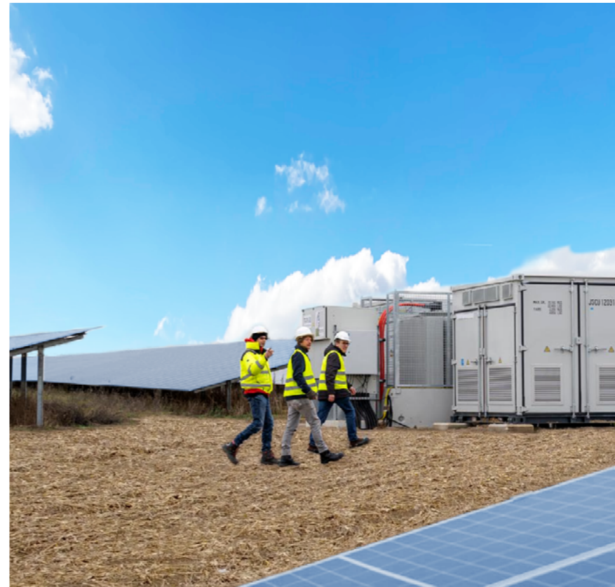
One of the largest PV plants in Germany with Sungrow inverters in Tramm-Göthen: 172 MWp with SG3125HV-20 plus 7.2 MV skid
